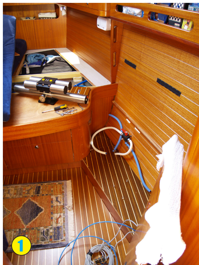
1. Installation is in the bow cabin. The small sofa has been taken apart to aid fitting. hoses have been positioned ready for the pressure intensifier & membrane
