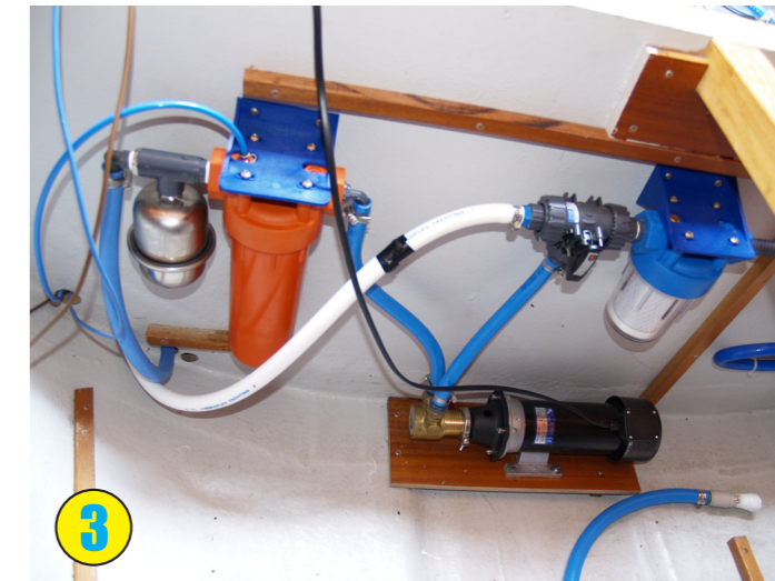
3. Filter assembly mounted on bulkhead, feed pump mounted below. All relevant hoses connected. Power supply connected.
