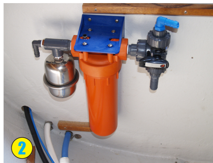
2. Filter assembly offered to the bulkhead to find the best position for easy filter change and service.
