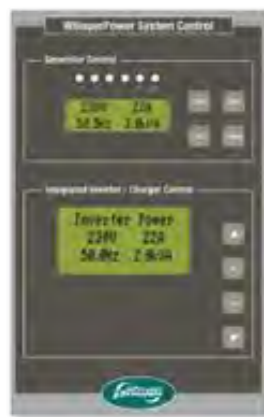
Genverter M-GV 7i Monitoring & Control panel: Generator Control (DDC), Extended Inverter / Charger Control + Ah Counting.
