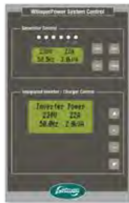
Genverter W-GV 7i Monitoring & Control panel: Generator Control (DDC), Extended Inverter / Charger Control + Ah Counting.
